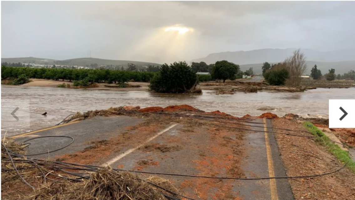
The Sinkhole on the R303 close to the Olifants River in Citrusdal. Picture: Tracey Adams/ ANA
